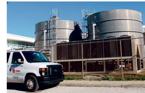
Over just the next five years, 63 schools need major A/C repairs or full replacements, 28 are in need of new roofs, and other schools have urgent needs to provide the right environment for teaching and learning.
