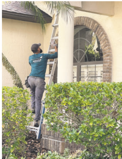
Vasquez goes up on the roof to inspect the raccoon entryway into the attic.
