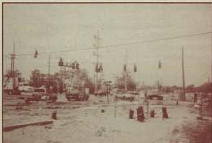
Construction along Bloomingtondale has progressed to the Bell Shoals intersection, where utilities are being replaced along the roadside.
