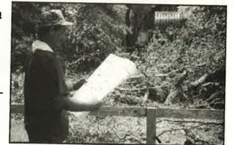
Site Foreman Calvin Hall monitors the necessary tree removal at the new YMCA site.
