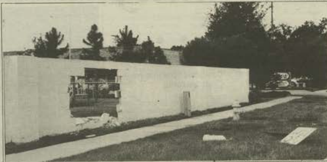
This hole in the wall could have had serious consequences if it had occurred during the week. A truck lost control and went through the masonry block wall that directly abuts KinderCare's outside play ground. Luckily, it was an early Saturday morning and no children were outside next to the wall.
