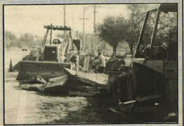
Crews lay ammonia pipeline as the work on widening Bloomingdale Ave. begins. Pipeline will be laid from Bell Shoals to John Moore and is expected to be completed by Christmas, after which road construction will begin.
