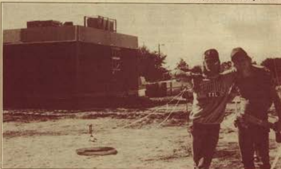
The construction on the new Mobil gas station at the corner of Bloomingdale and Bell Shoals is almost complete as seen by the happy grins on the gentlemen doing the work. Contrary to popular belief, this Mobil station is not owned by Bill Bradley, who owns the other Mobil station less than one mile away at the corner of Kings Ave. and Bloomingdale. Needless to say, Mr. Bradley is not very pleased with Mobil's decision to put a corporate station so close to his own.
