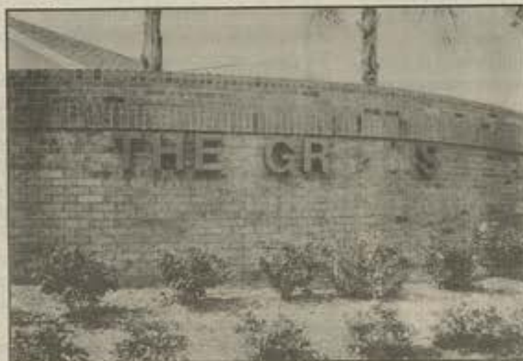
Brass letters on entry signs are a common target for vandals. They cost approximately $50 to $75 each to replace.
