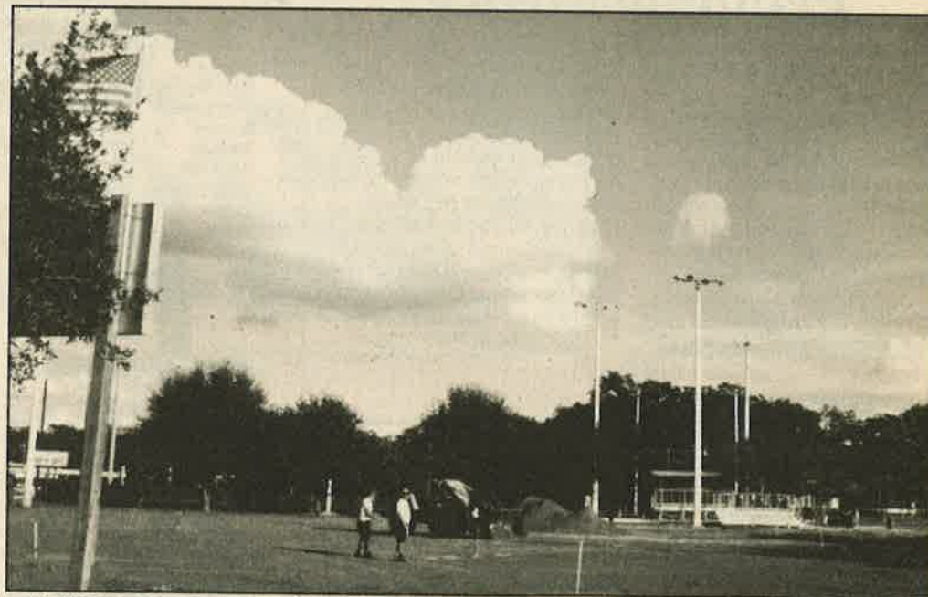
All South Baseball, Inc. contractors Guy Sheppard and Robert Rose start laying the clay for the new Major field infield. The company has completed several of the new projects at Bloomington Little League Park.
