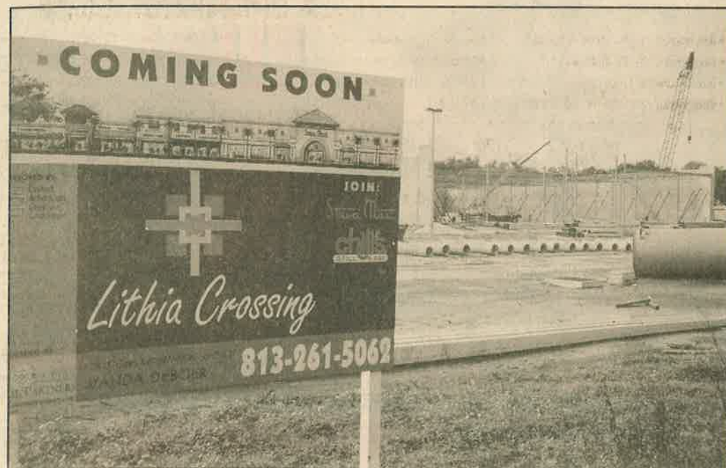
The construction of Lithia Crossings Shopping Plaza on Lithia-Pinecrest Road is well underway. Many residents say new shopping and dining destinations convenient to our area are welcome additions, but on the flip side, they are sure to result in more traffic congestion.
