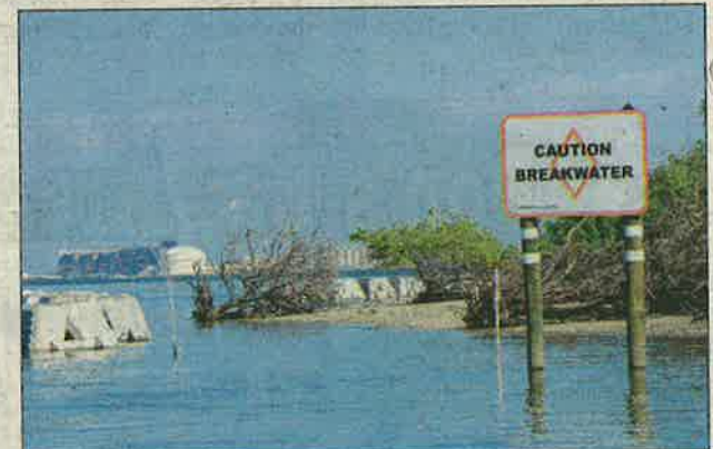
Toppled trees on the Sunken Island beach illustrate why Audubon of Florida installed a series of custom-concrete structures to try to shore up the island, a prime Tampa Bay nesting site for up to 18 species of birds.
