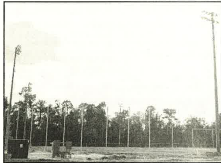
The first phase of the Campo Family YMCA, the construction of a new senior baseball field next to the new facility, is in its final steps. The lights are up, the clay is down, the fence is being installed, and the parking lot is ready for paving. It won't be long before the real sounds and signs of spring are in the air. The new field will be tremendously welcomed by the many players at Bloomingdale Little League. Photo by Mack Austin.
