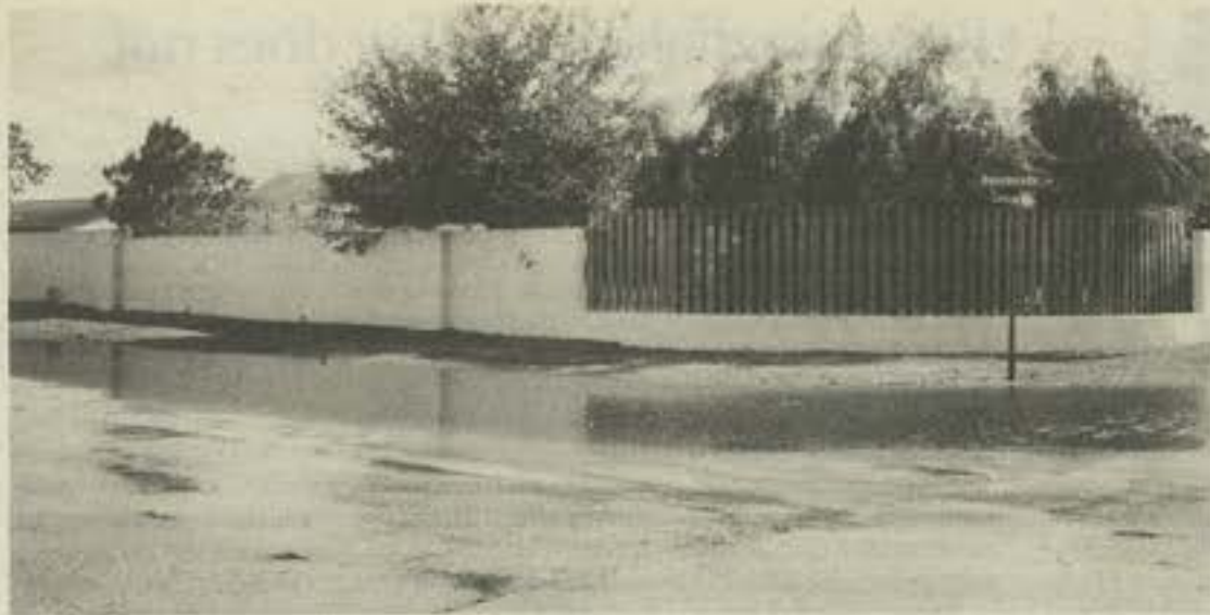
A water main split Feb. 22 at the intersection of Rosemead Lane and Canoga Park Drive in Bloomingdale, sending underground water onto the north, south and western roadways. Jack Dempsey, utility maintenance supervisor of Hillsborough County's Public Utilities Dept., said moisture and a shifting terrain were responsible for the damage. The incident was unrelated to a storm drain split that occurred two days earlier two blocks away, Dempsey said.
