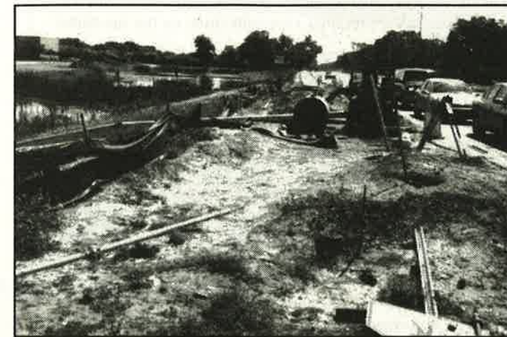
Construction on Bloomingdale Avenue has been delayed. The County now estimates an August completion date.
