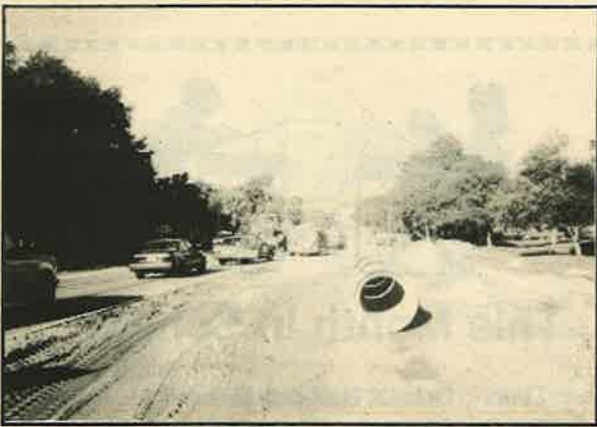
County officials say road widening on Bloomingdale from John Moore to Bell Shoals is right on schedule. Extensive work has backed up motorists mornings and afternoons as far as east of Bryan Road.
