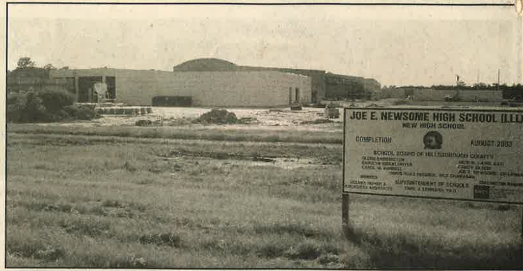
Construction is progressing on Newsome High School on Fish Hawk Boulevard in Lithia. MACK AUSTIN/Photo
